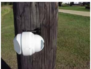
Driveway in upper right hand corner of this picture shows another angle of the behind the pole mount V bracket.
